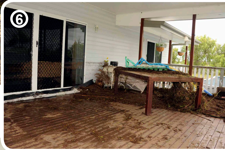
Below: Residential property flood damage and debris.
