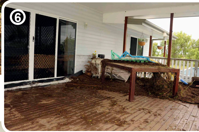
Below: Residential property flood damage and debris.
