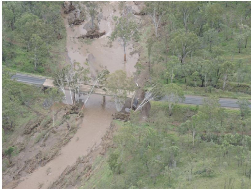
Figure 4-22 Eroded abutment of the Dawson Highway bridge over Callide Creek
